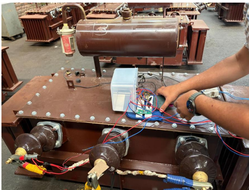
Figure: Hardware prototype ESP32 microcontroller with sensors mounted on a distribution transformer at the manufacturing facility. Wires connected to HV/LV bushings for real-time current, voltage, temperature, and vibration measurement.
